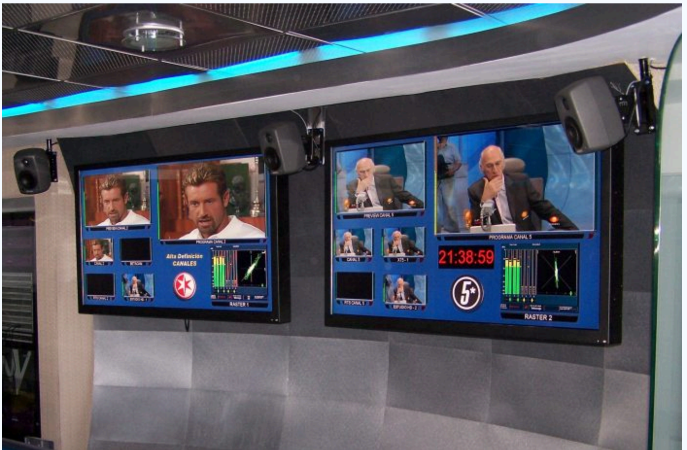
Multimage Monitor Wall built with SPARROWHAWK LSM 157W
