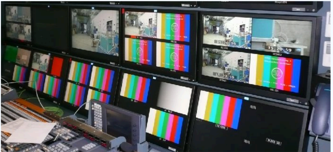
Customized Monitor Wall in an OB truck built with BLACK MILAN QLM 124W and SPARROWHAWK LSM 124W HD
